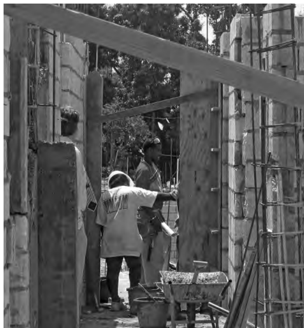
Grants Pen resident and laborer help with construction of the new multipurpose facility.
