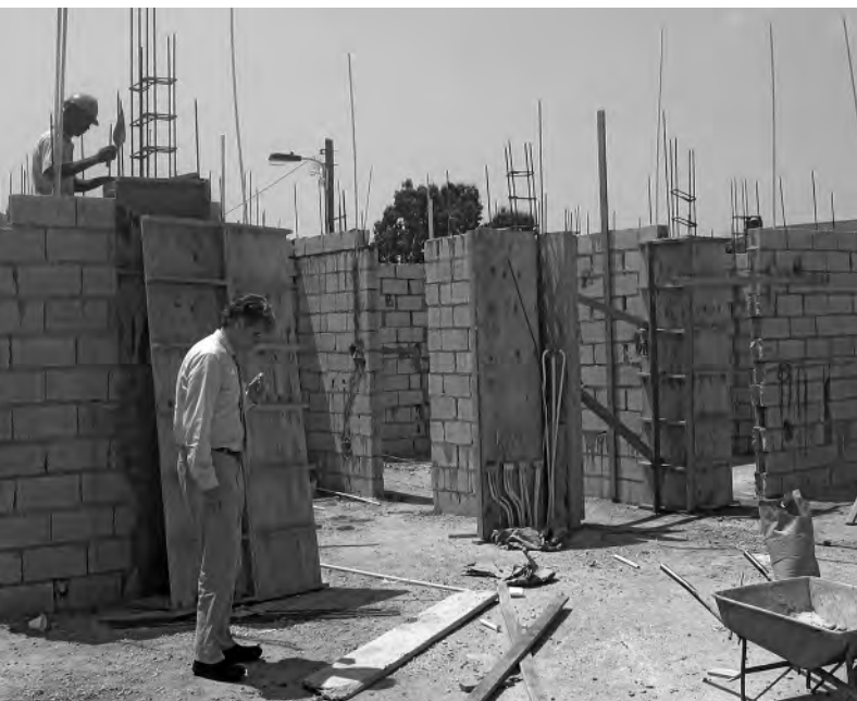
PERF Consultant William Andrews observes construction progress at the site of the multipurpose facility.
