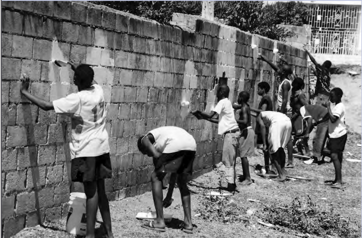
Grants Pen community members paint a wall during a community improvement project.
